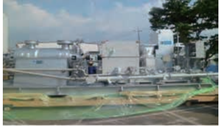
Turbine driven (2sets)
