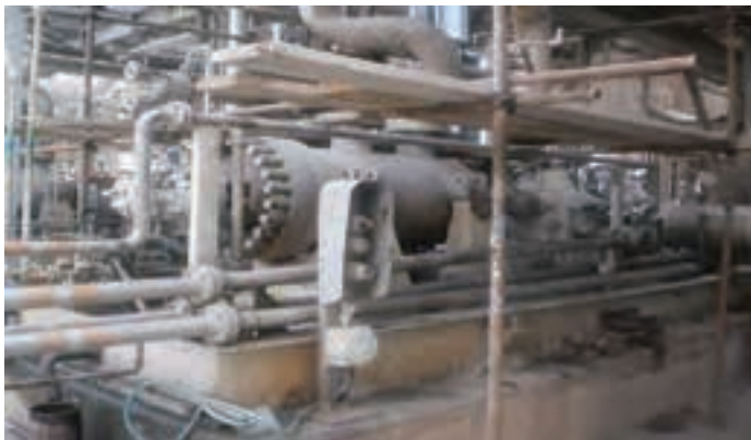
Existing pump (PIGONE, ITALY)
